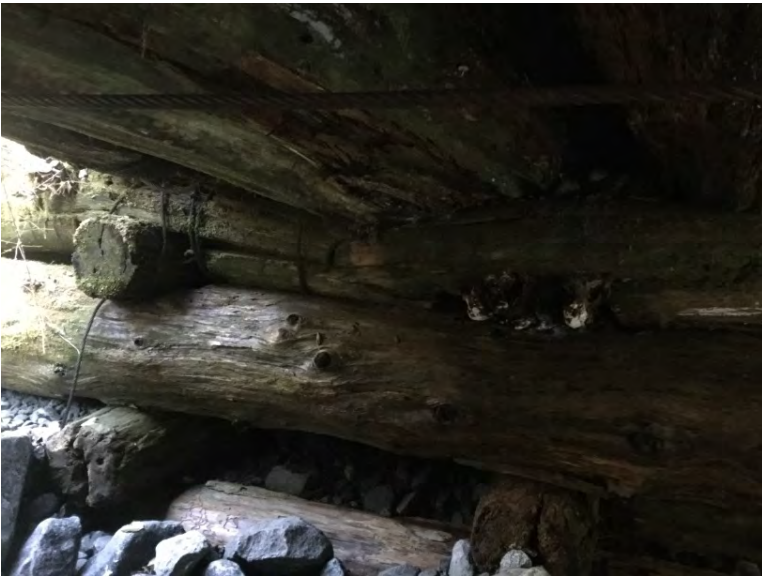
Top crib log at left bank cracked horizontally and vertically
